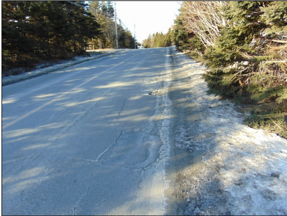
Figure 20: Asphalt condition on Snow's Lane
